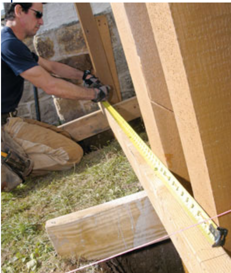
Figure 4. The author lays out the post locations on a 2-by that will also be used to align and brace the tops of the posts.
