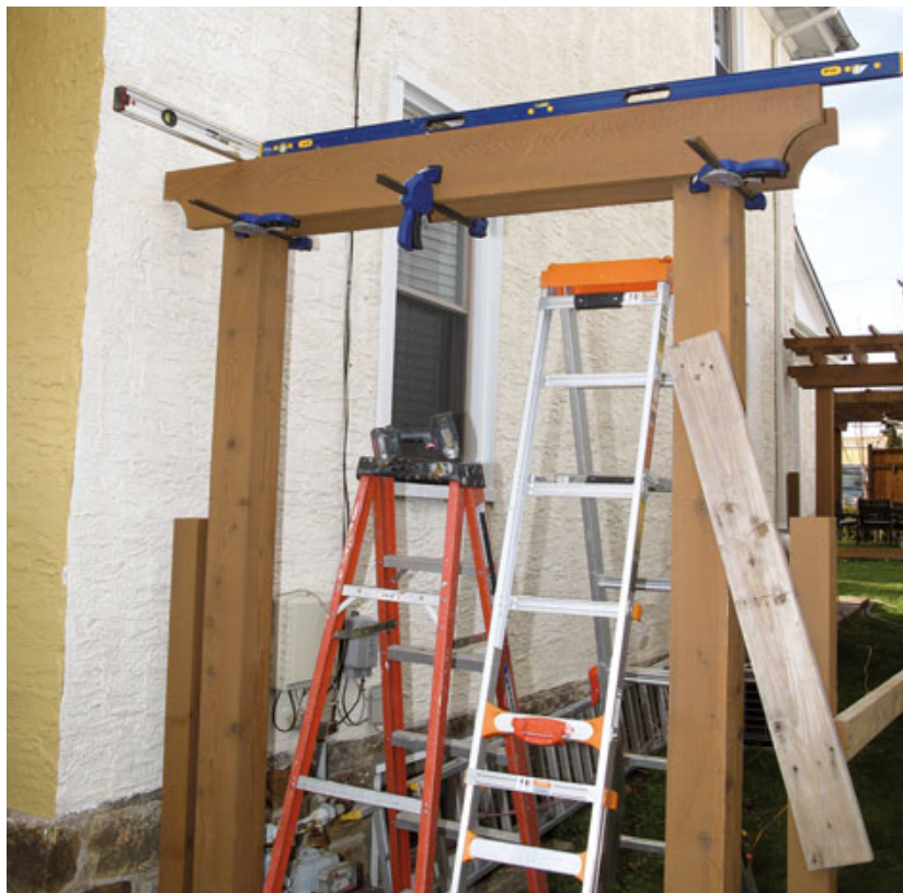
Figure 5. Temporary bracing holds the posts in place until the framing is complete.
