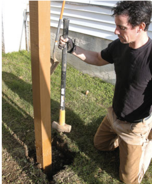
Figure 3. The bottoms of the posts rest on gravel for drainage and are topped with a bag of quick-setting concrete to keep them steady. Tamping the soil adds more stability and minimizes settling.
