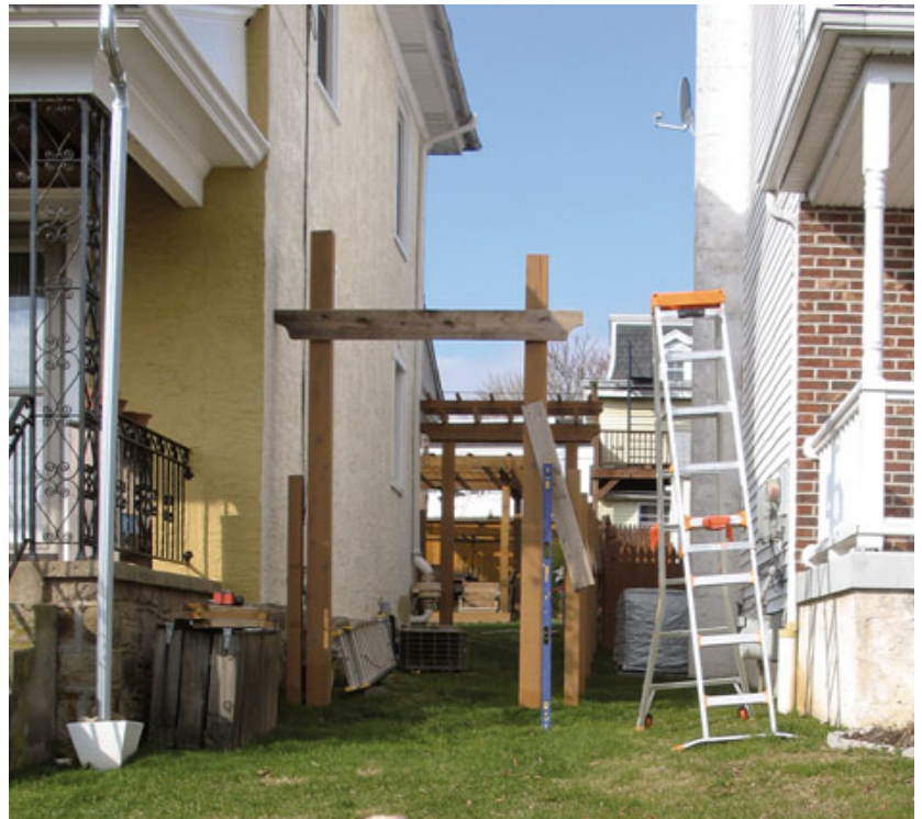
Figure 2. Full-size mockups of the girder and other parts were used to verify that the proportions looked right.
